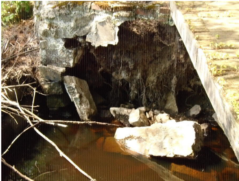
Collapsed left training wall of the auxiliary spillway at the Home Brew Dam.
