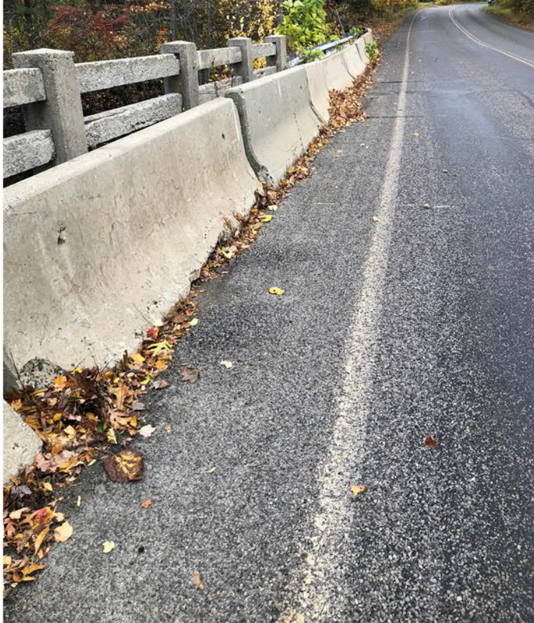
Jersey barriers at the crossing upstream of the dam at 371 Aldrich Street.
