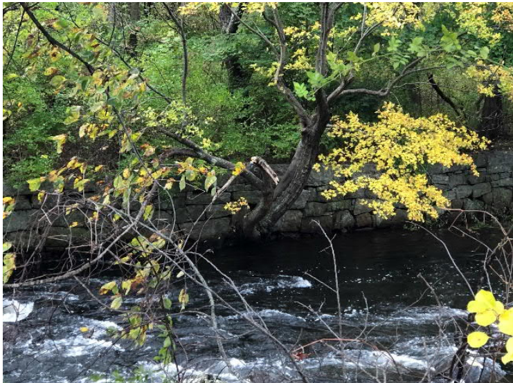
Tree growth through a training wall at Whitin Pond Dam.
