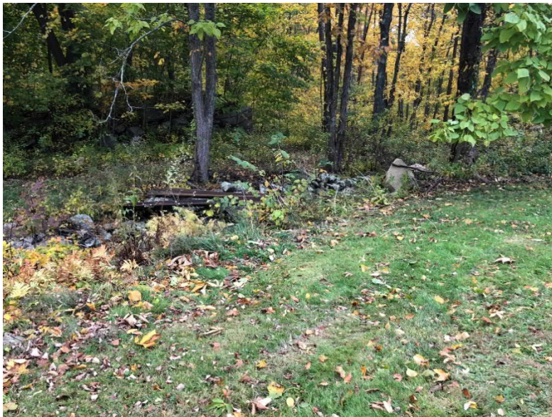
Trees growing on the embankment of the dam at 371 Aldrich Street.
