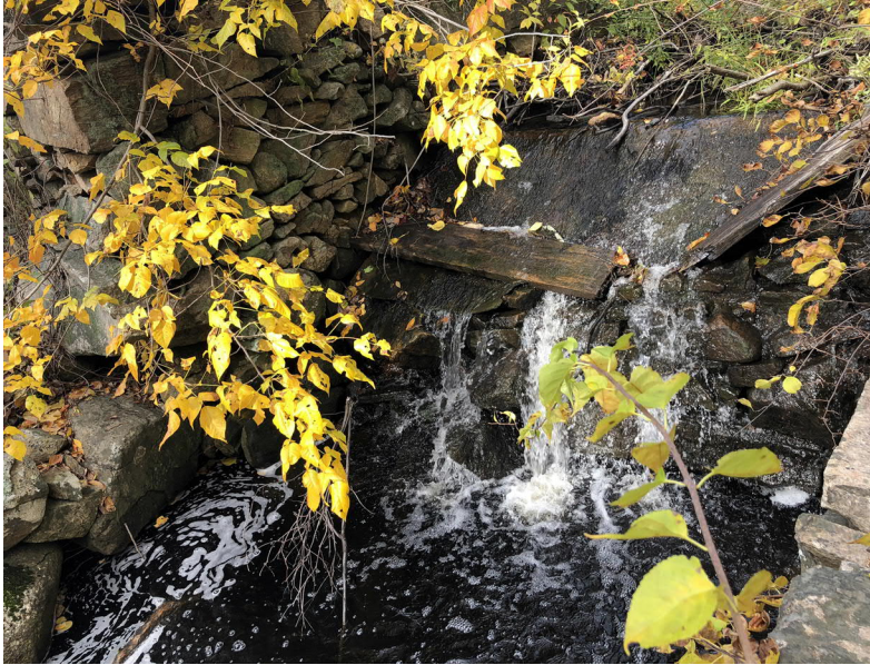
Spillway of dam at 371 Aldrich Street. Note broken weir boards and voids in the spillway and training walls.
