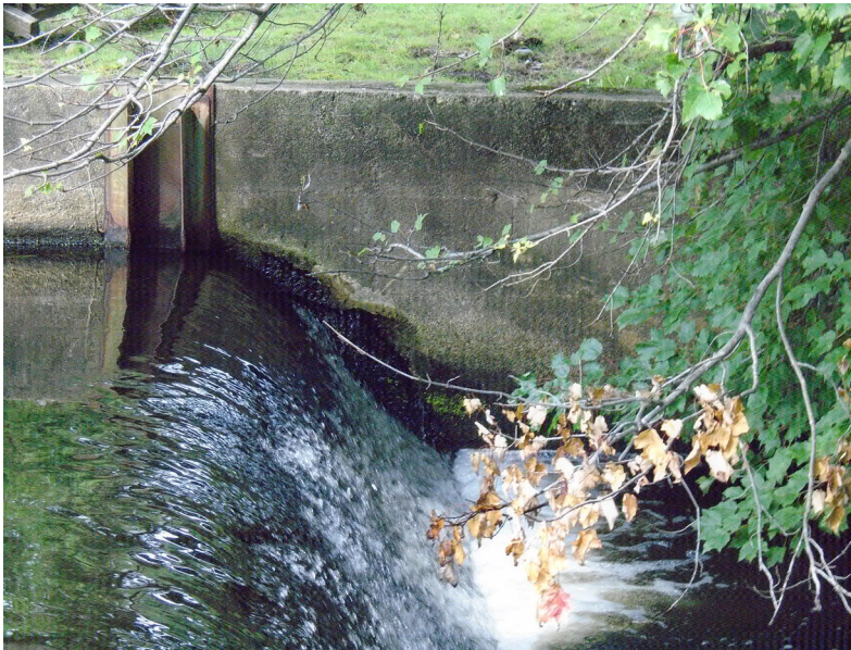
Left training wall at Ironstone Reservoir Dam. Note the seepage along the training wall just above the spillway.
