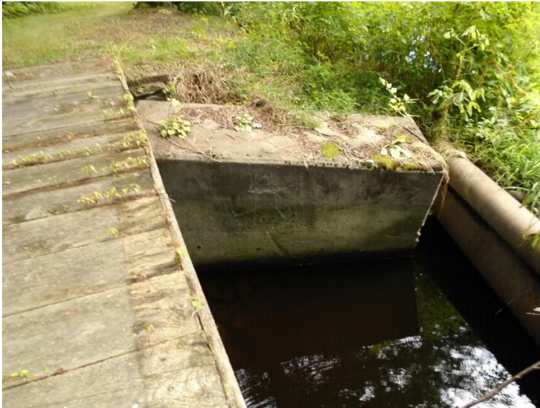
Separation of the right training wall of the auxiliary spillway from the right abutment of the Home Brew Dam.
