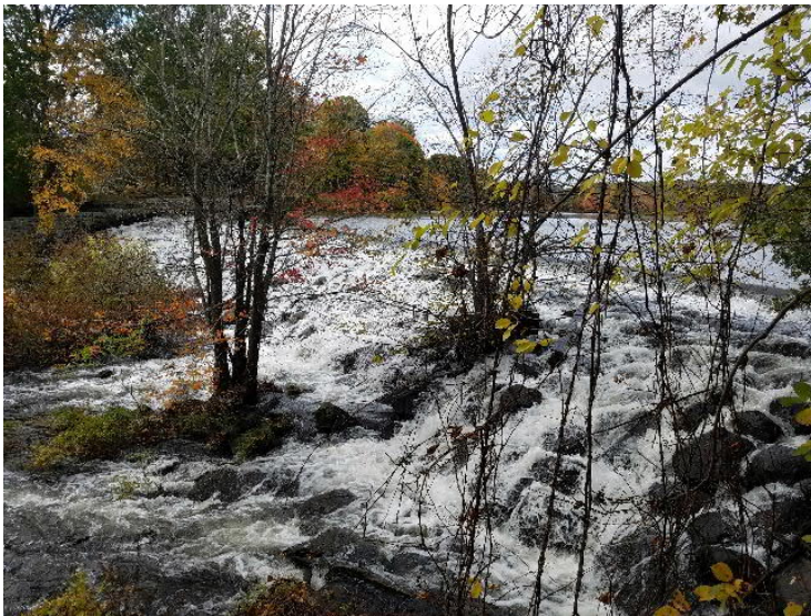
Primary spillway at Whitin Pond Dam. Note the growth of trees and woody vegetation in the spillway.
