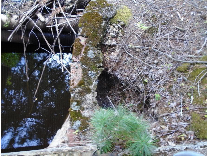
Sinkhole behind the left training wall of the auxiliary spillway at the Home Brew Dam.
