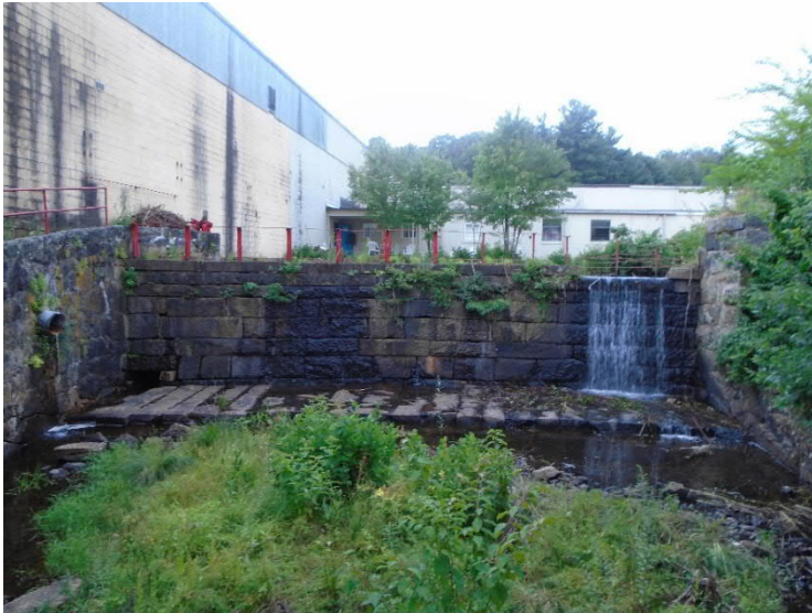
Rivulet Village Pond Dam spillway. Note the vegetation growing through the walls and downstream face of the spillway.
