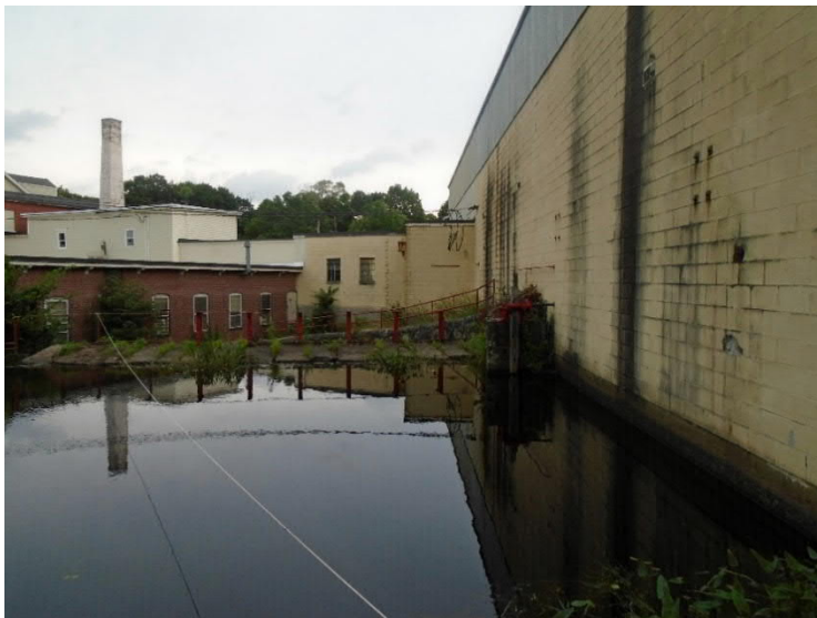
View facing downstream at the Rivulet Village Pond Dam spillway from the impoundment. The mill building has flooded multiple times during high flow events.
