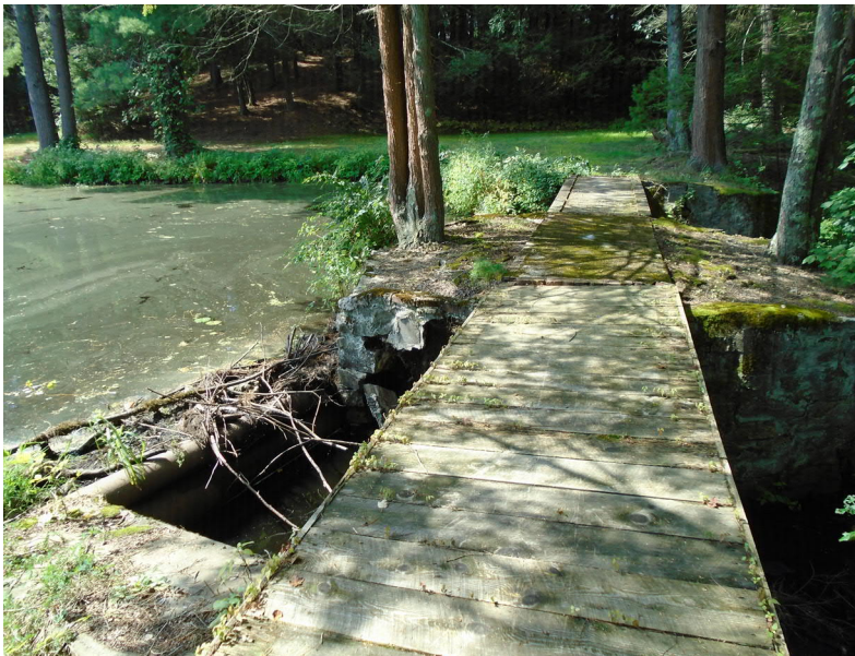
View of the Home Brew Dam from the right abutment. Note the debris accumulated behind the pipes immediately upstream of the auxiliary spillway and the collapsed left training wall of the auxiliary spillway.
