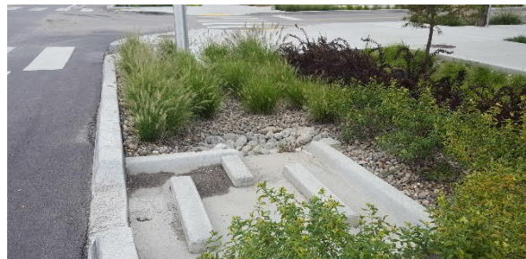
Image 1: Example of an established bioretention basin with a concrete curb cut and concrete pretreatment structure to remove sediment before runoff enters the planted portion of the basin. Image source: Fuss & O'Neill
