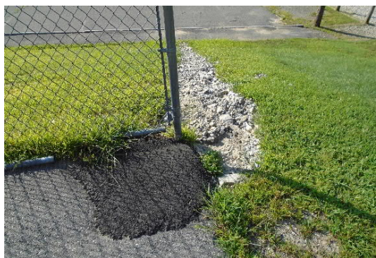
Image 2: Armored swale and a damaged portion of the basketball court due to concentrated stormwater runoff. Image source: Fuss & O'Neill
