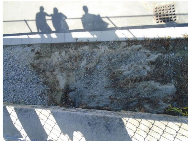
Image 3: Sediment deposited below an area of seepage through the retaining wall between the fire station and Park Street. The seepage flows at extremely high flow rates during rain events and appears to be associated with the catch basin in Image 2 (which is also located just outside the bottom edge of this image).
