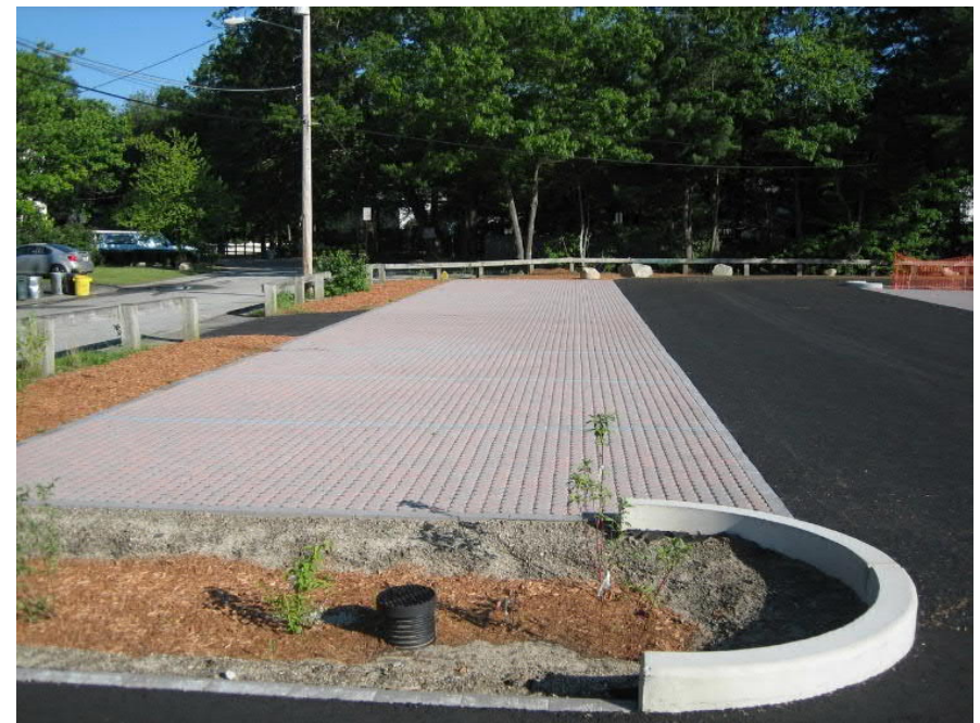
Image 3: Permeable pavers installed in parking spaces within a parking lot. Image Source: GeoSyntec
