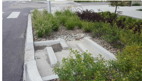
Image 1: Example of an established bioretention basin with a concrete curb cut and concrete pretreatment structure to remove sediment before runoff enters the planted portion of the basin. Image source: Fuss & O'Neill
