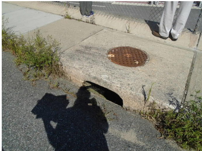
Image 2: A catch basin on Park Street that appears to be associated with flowing seepage through the adjacent retaining wall (see Image 3).
