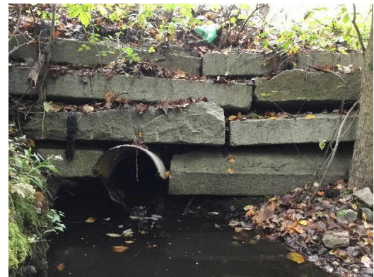
Figure 21. The outlet at the crossing on Albee Road (xy42040747159721). Note the misalignment of the stone blocks forming the culvert endwall.
