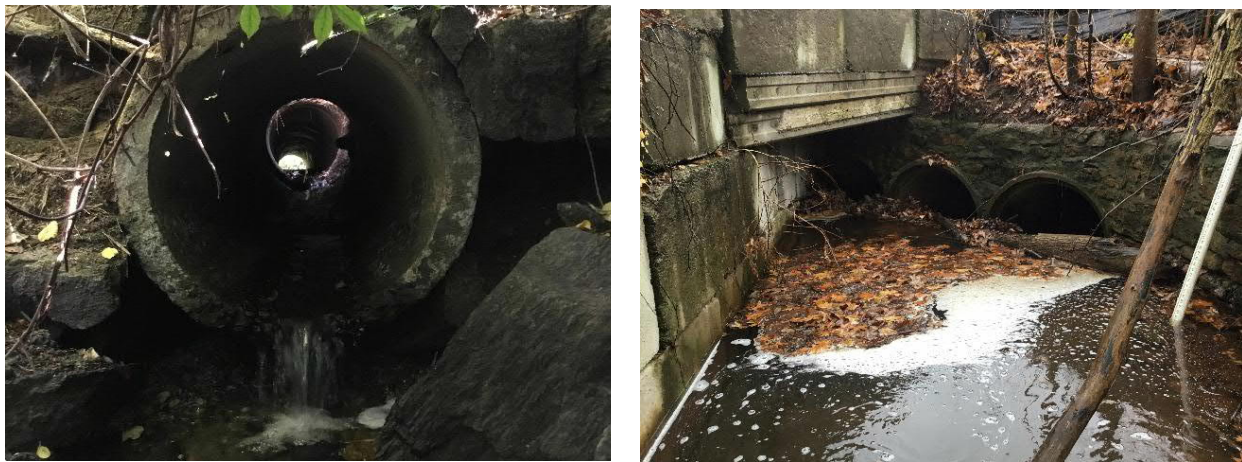
Figure 2. Examples of crossing structures in poor structural condition observed at various locations during field assessments. Left: Structure exhibiting a sinkhole, critical structural integrity, and critical joints and seams. Right: Severely blocked culvert inlets.
