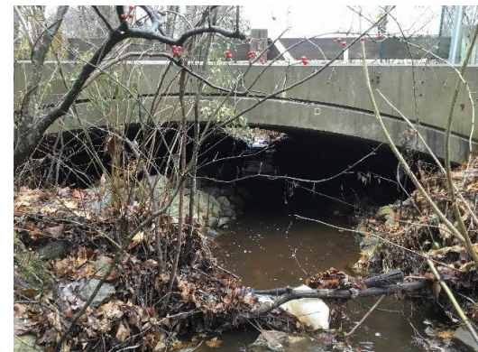
Figure 19. The outlet at the crossing on Taft Hill Lane (xy42069427166042). Note the accumulation of debris on banks that appear to have been incorrectly constructed within the crossing.
