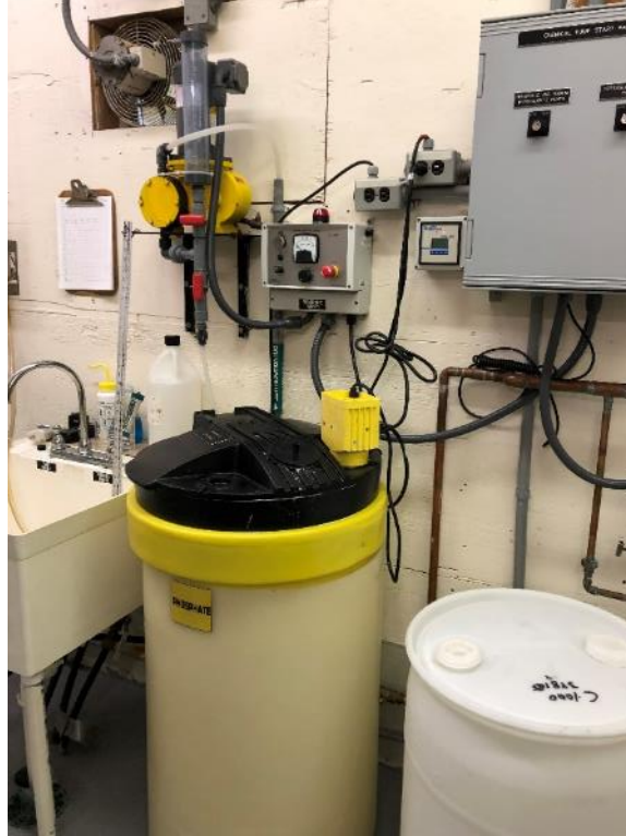
Figure 3-8. Phosphate Chemical Feed System
