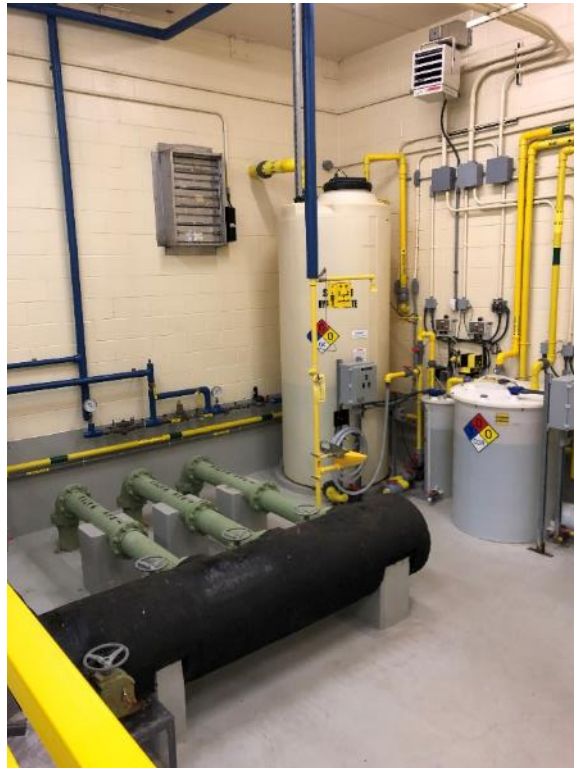
Figure 3-19. Sodium Hypochlorite Feed System
