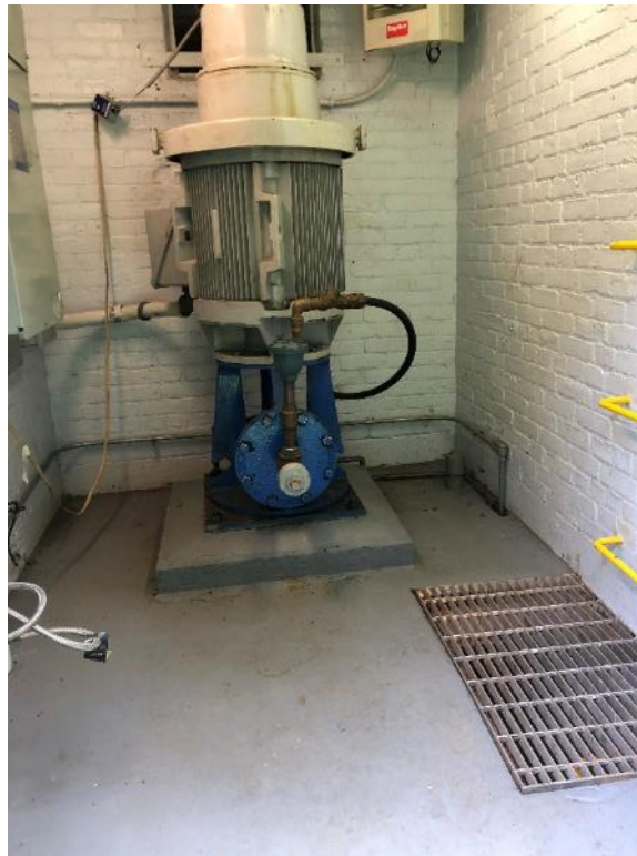
Figure 3-10. Bernat Well Pump Station
