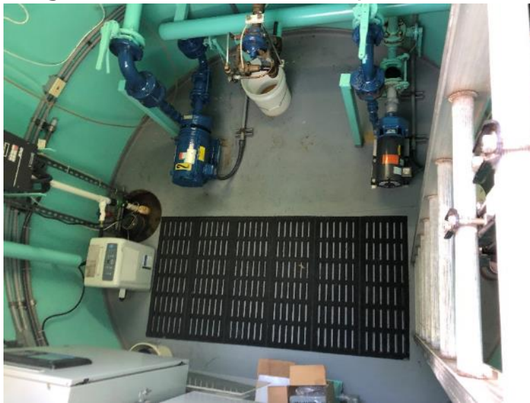
Figure 3-22. East Street Booster Pump Station Interior
