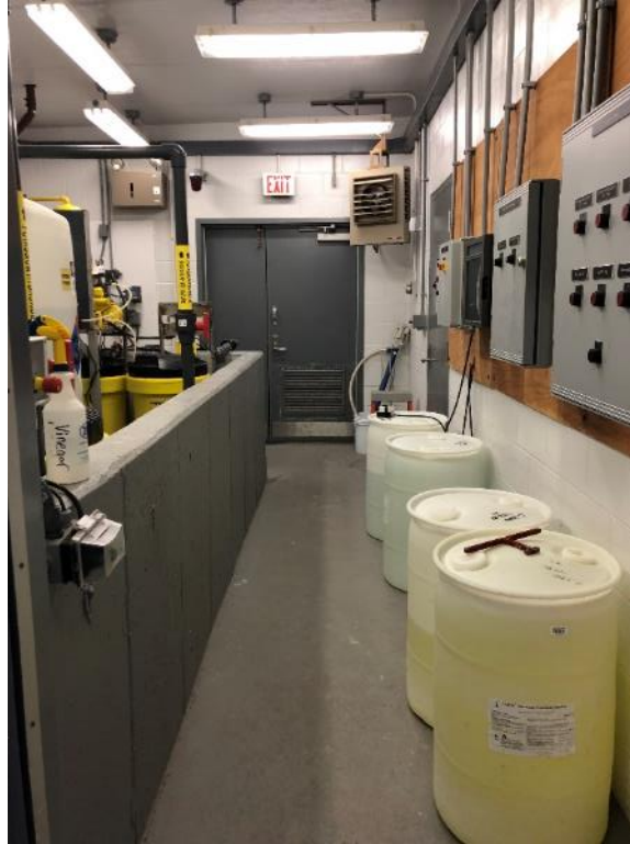
Figure 3-13. Bernat Chemical Feed Room
