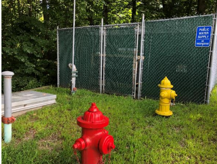
Figure 3-21. East Street Booster Pump Station Exterior
