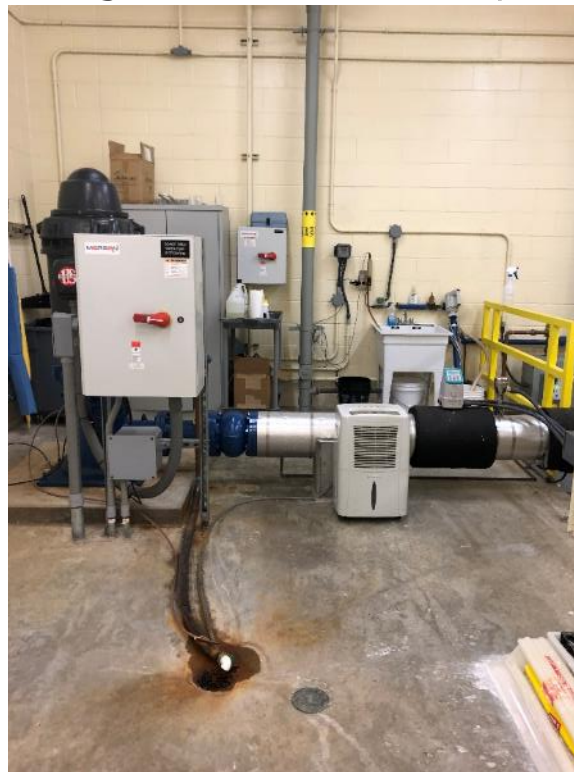
Figure 3-17. Rosenfeld Well Pump
