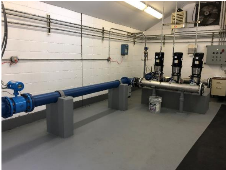
Figure 3-24. Farfard Booster Pump Station Interior
